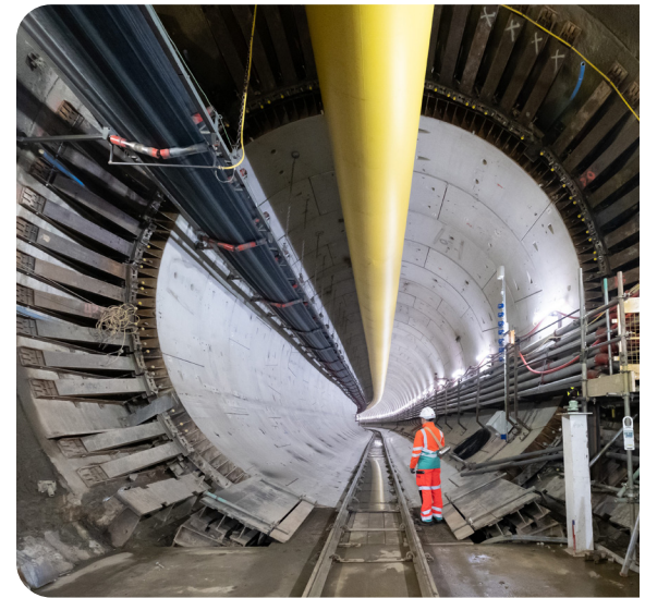
The Thames Tideway Tunnel is now operational and will reduce the volume of discharges into the tidal Thames by around 95% leaving behind a cleaner, healthier river
