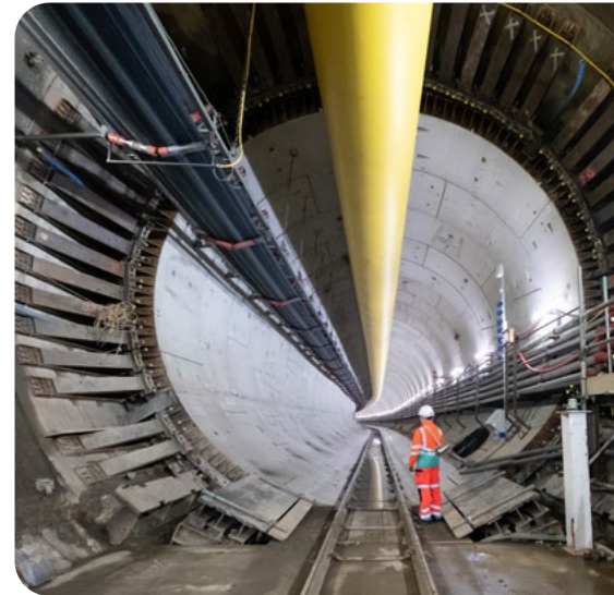
The Thames Tideway Tunnel is now operational and will reduce the volume of discharges into the tidal Thames by around 95% leaving behind a cleaner, healthier river
